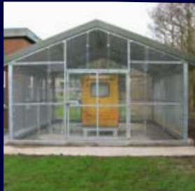
Generator housing Garstang
